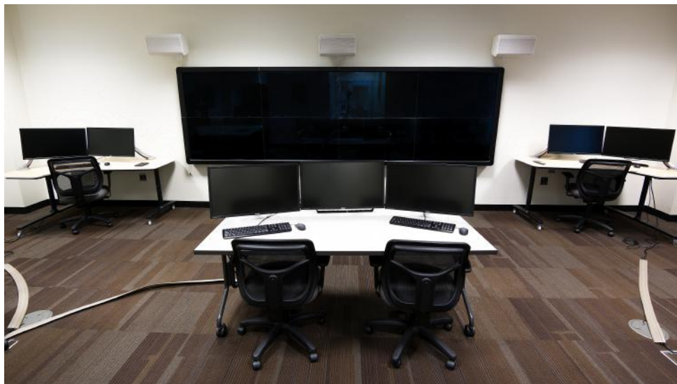
Figure 2. ACES Installation in PKI, 335
